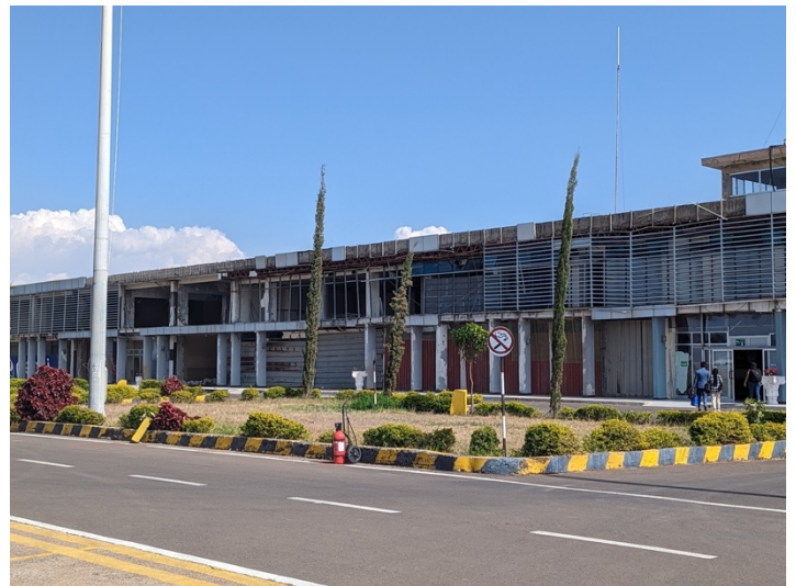
Figure 1 - Explosion damage to the airport terminal is visible caused by rebels attempting to disable the airport in Bahir Dar
