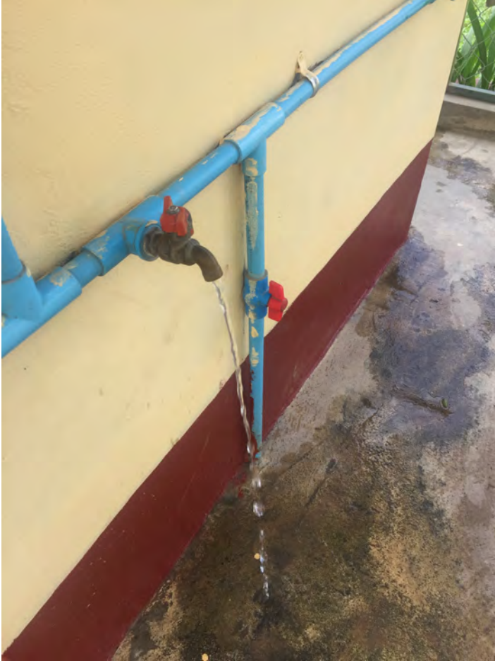
Clean water exiting the filter.
